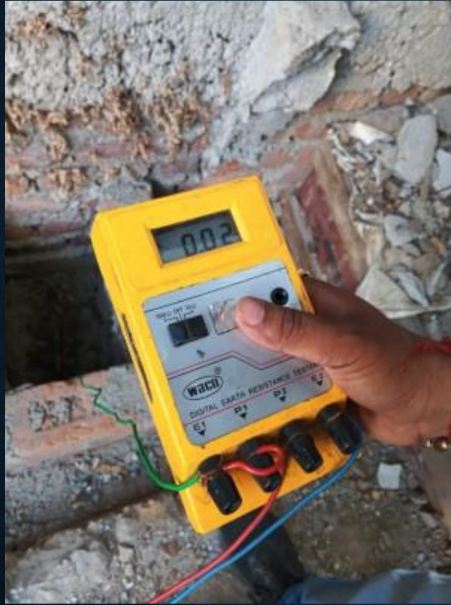
Digital Earthing Testing
